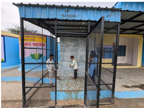
Rain Water Harvesting System (1,00,000 litres)
